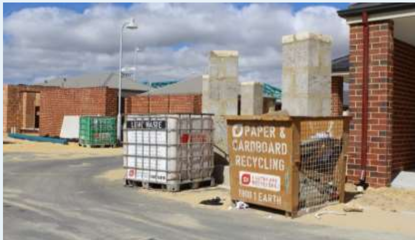
Figure 4: Source separated waste destined for recycling at a residential construction site in Perth
